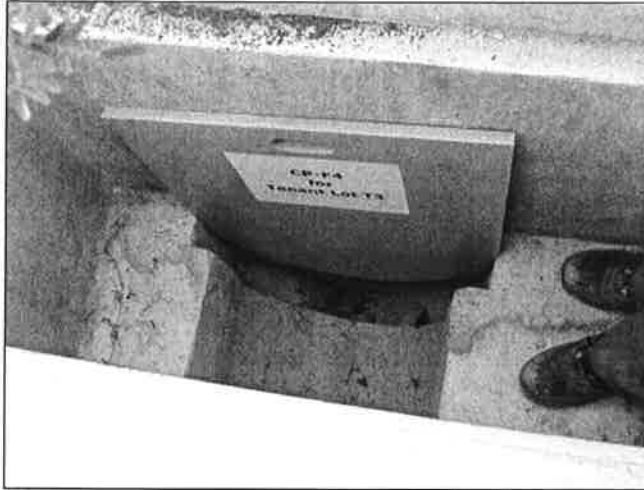
Figure 8-3 Stop-log in Place in Lot Occupied by Tenancy EP06-033 (2 of 2)
